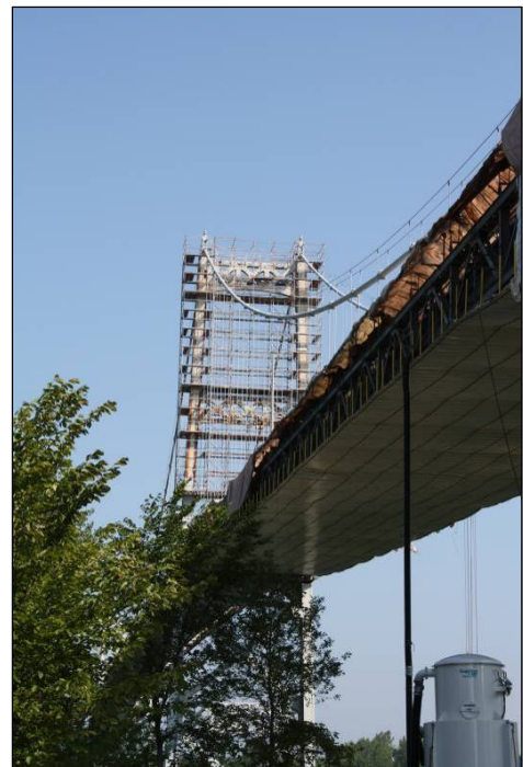
View from U.S. viaduct of scaffolding and work areas for Phases 1 and 2 of the Seaway International Bridge recoating project.
