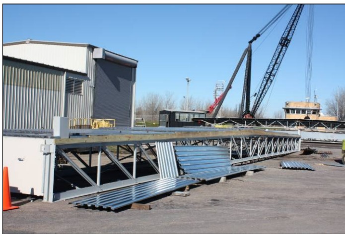
Newly refurbished and insulated lock covers will provide better lock access during winter work and save lock chamber heating costs.
