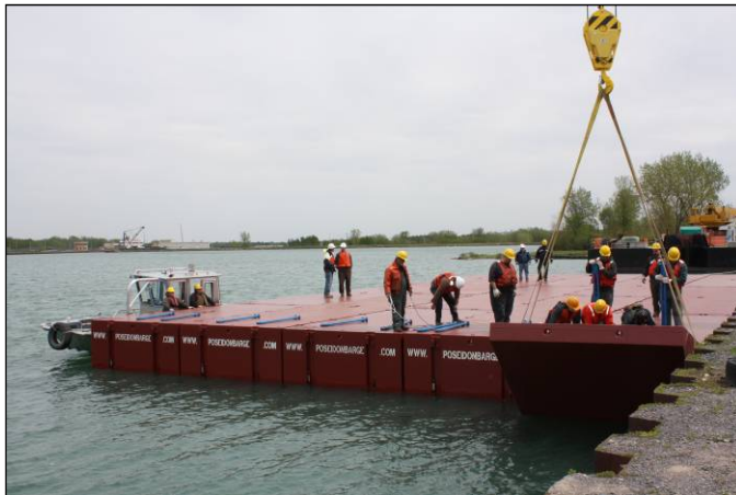
Corporation personnel, under the direction of Poseidon Barge Corp. representatives, are assembling the sectional spud barge for the first time.
