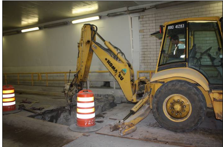
Contractor removed concrete to expose joints below roadway surface for grouting and sealing.
